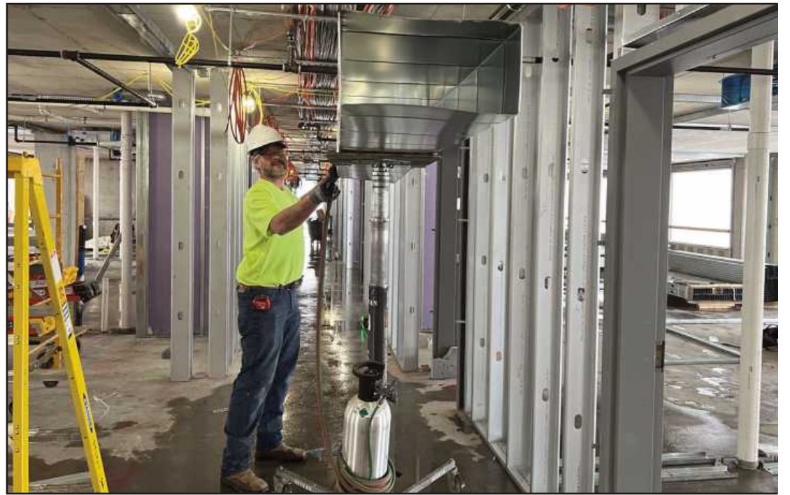
LIFTING A DUCT into place on the sixth floor at the Vanguard Hotel project in Ann Arbor is Rob Liedel III of Sheet Metal Workers Local 80. He is employed by Sylvan.
