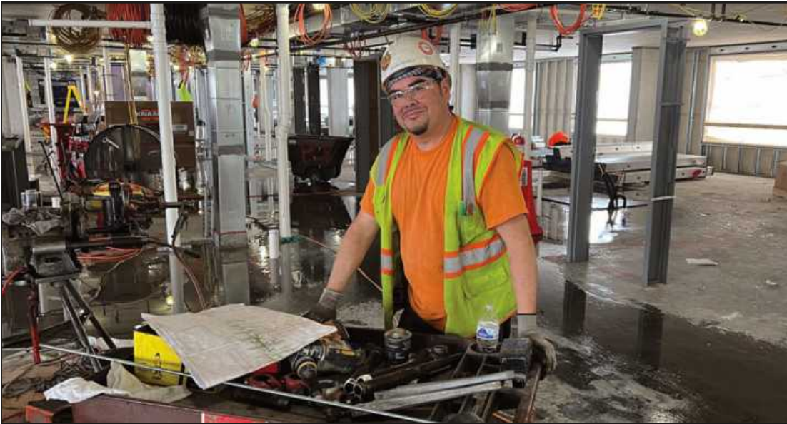
AT WORK ON THE sixth floor of the Vanguard Hotel project in Ann Arbor is Michael Escamilla of Sprinkler Fitters Local 704. He's employed by VFP Fire Systems.
