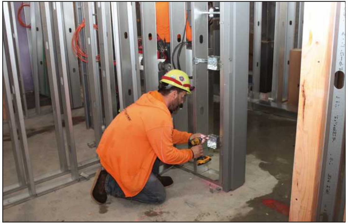
SETTING A BOX in what will be a guest room at the Vanguard Hotel project in Ann Arbor is electrician Mike Sherwood. The IBEW Local 252 member is employed by Superior Electric.
