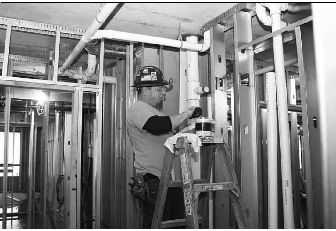
SETTING A WASTE VENT in a fifth floor room at the Vanguard Hotel in Ann Arbor is Chris Young of Plumbers and Pipe Fitters Local 190. He's employed by Wilbur Plumbing.
