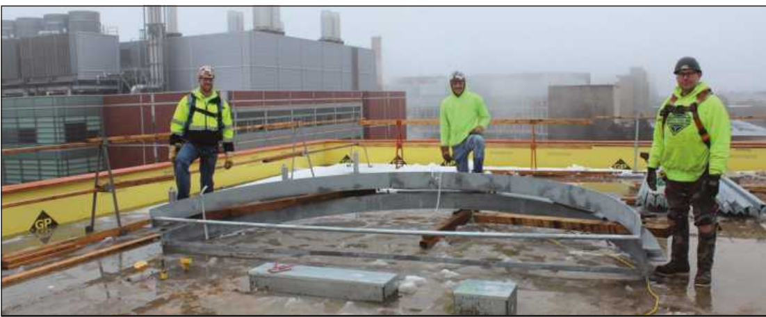
WE ASKED THIS TRIO of iron workers to gather 'round the "oculus" – an architectural element they're building on the foggy roof of the Vanguard Hotel project in Ann Arbor. From (l-r) are Ken St. Louis, Brandon DeBord and Mark James. The Local 25 members are employed by Vertex Steel.
