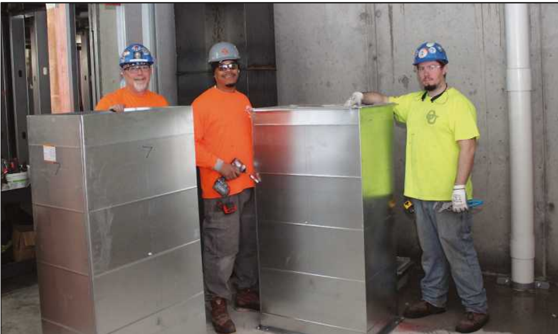
SETTING UP SUPPLY ducts on the fifth floor of the Vanguard Hotel project in Ann Arbor are (l-r) Jeremy Jundro, Lawrence Cochrane and Anthony Nastwold. The Sheet Metal Workers Local 80 members are employed by Sylvan.
