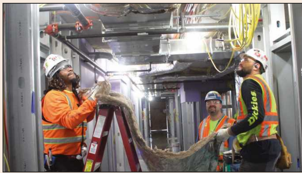
UNDER THE WATCHFUL EYE of foreman Tim Wood II, first-year apprentices (l-r) Rodney Ambrose and T.J. Caudill insulate a duct in a fourth-floor hallway of the Vanguard Hotel project in Ann Arbor. The Heat and Frost Local 25 members are employed by Master Mechanical Insulation.
