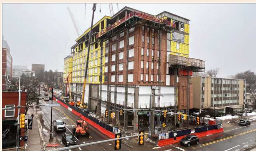
THE VANGUARD HOTEL under construction at Catherine between Glen and Ann streets in the Ann Arbor Medical Center fills a need for the area, with the addition of 164 hotel rooms. Colasanti is managing the project, and about 115 tradespeople are on site.
