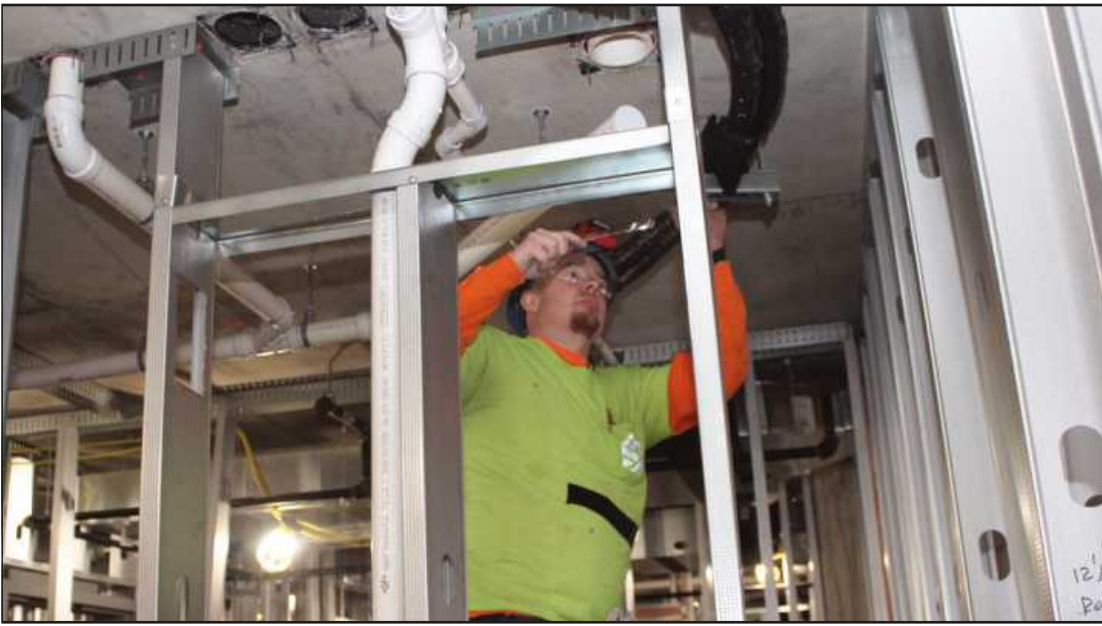
RUNNING HEATING and cooling pipe on the fifth floor of the Vanguard Hotel in Ann Arbor is Paul Dancy of Pipe Fitters Local 636. He's employed by Sylvan.
