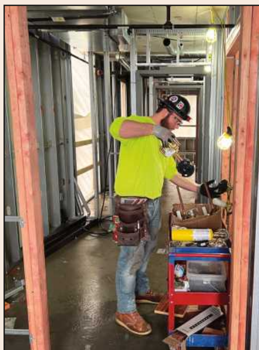
SETTING UP A SHOWER valve for installation in a sixth floor room at the Vanguard Hotel project is Eric Kinney of Plumbers and Pipe Fitters Local 190. He's employed by Wilbur Plumbing.
